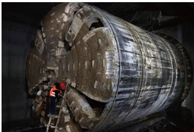
Figure 1 (Color online) A clogged cutterhead after excavation.
