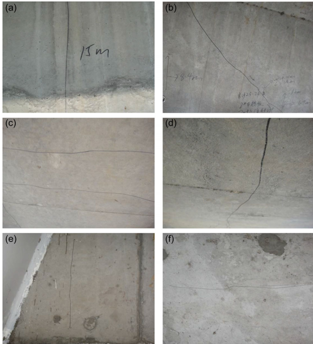
Figure 13 (Color online) Typical types of cracks of Xinyihe Bridge. (a) Vertical web crack; (b) diagonal web crack; (c) transverse crack at girder bottom; (d) longitudinal crack at girder bottom; (e) vertical crack at the end of crossgirder; (f) transverse wet joint crack.
