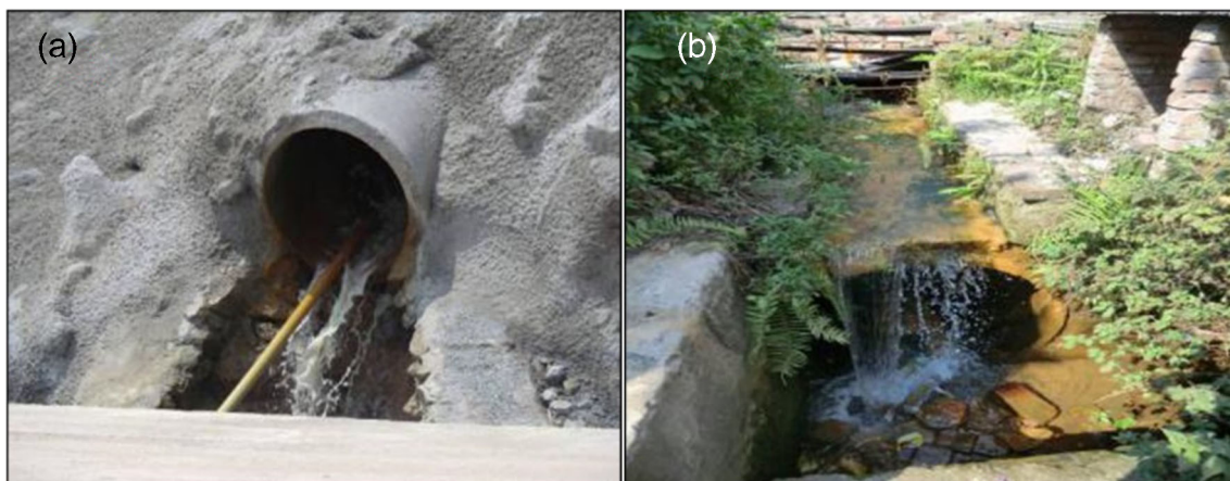
Fig. 2 The groundwater drainage forms of (a) pipeline and (b) Ditch during the tunnel excavation
