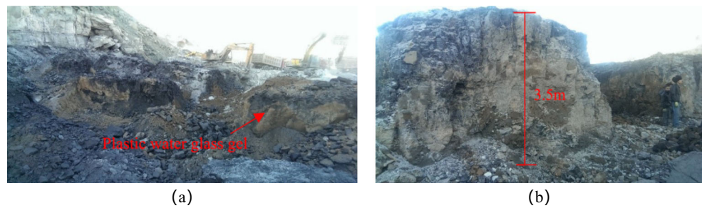
Fig. 16 Stripping construction site: (a) plastic sodium silicate gel almost filled the entire goaf, and (b) the height of the water-glass gel stack can reach the top of the A2 coal seam
