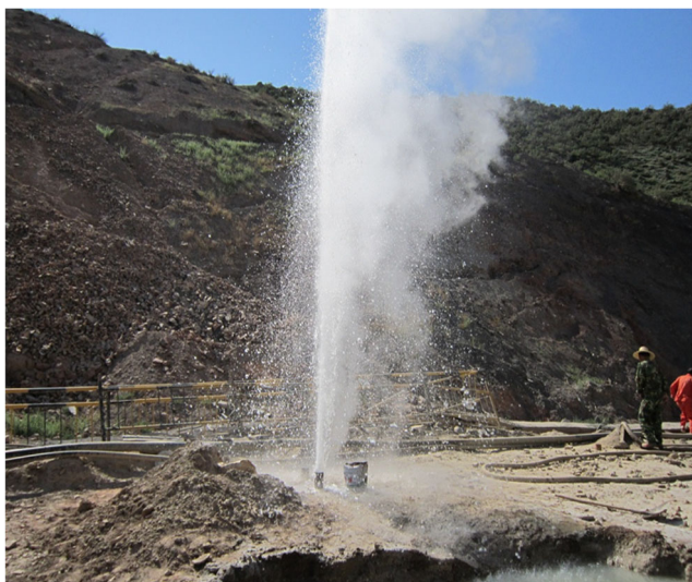
Fig. 14 Water column produced during grouting (due to the high temperature in the borehole, part of the slurry rapidly vaporizes, resulting in slurry jetting out of the borehole and forming a 10-m-high water column)
