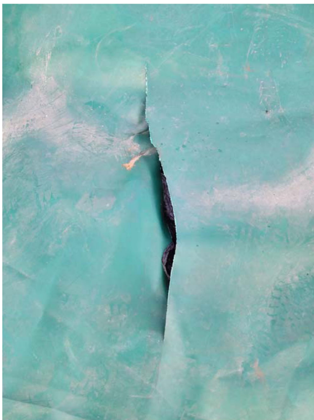
Fig. 6 Defects on temporary HDPE cover at the landfill site
