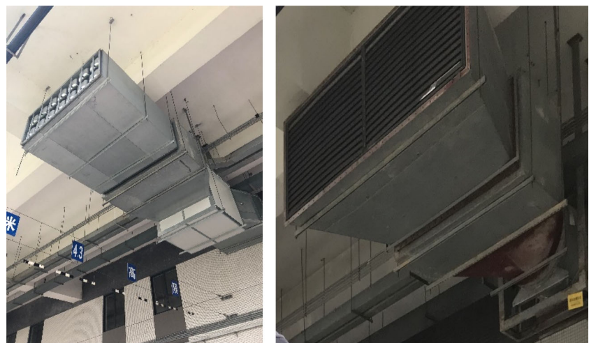
(a) Ventilation fan with silencer
