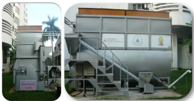
Fig. 2 Configuration of the developed prototype single-stage anaerobic digester for conversion of food wastes to biogas
