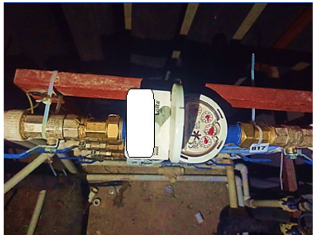
Fig. 10 The end-device (water-meter) installed in the elevator shaft of the building
