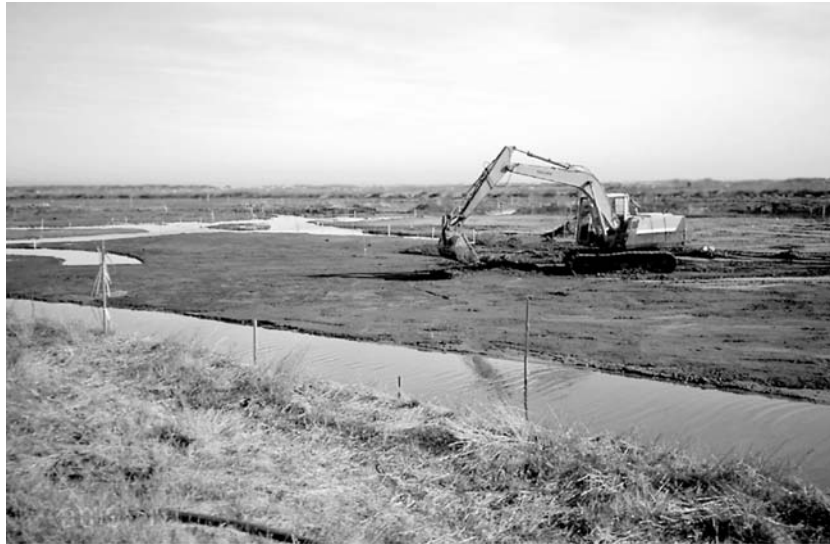
Figure 3. Excavation of sediments to restore an 8-ha marsh at Tijuana Estuary, San Diego county, CA. Excavation was designed to set up a large field experiment. On the left is one of three replicate marsh-plain areas having tidal creeks; on the right is one of three marsh-plain areas without tidal creeks.
