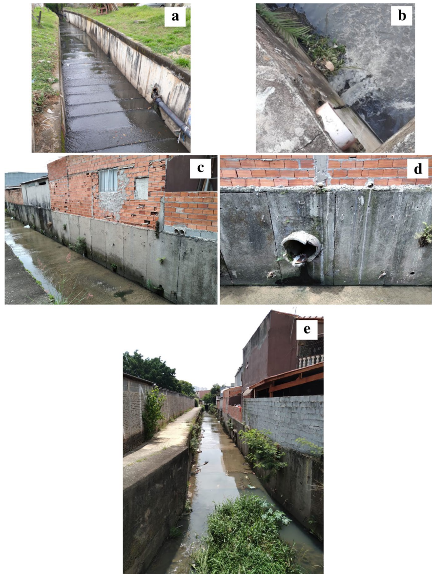
Fig. 2 Current condition of Comprido stream: a channeled bed; b , c , and d examples of domestic sewage discharges along the water body; e example of building in the banks of the stream. Source: authors
