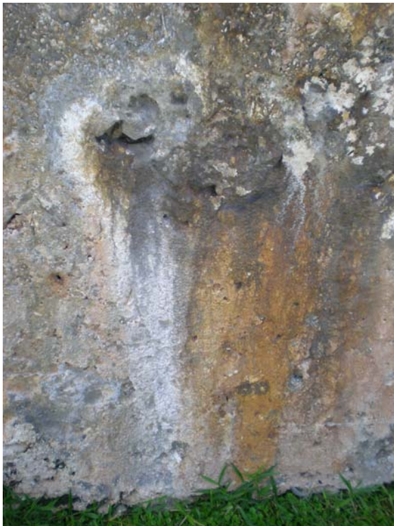
Fig. 11 Example of Carsick structures provoked by water infiltration observed at San Pedro and San Carlos fortress
