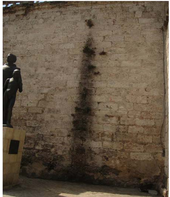
Fig. 9 Basilica Minor San Francisco de Asis, San Francisco Square wall. Patina formed due to water drainage
