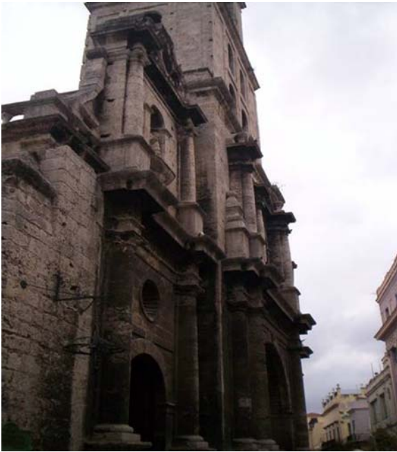
Fig. 7 Facade of Basilica Minor at Oficios Street. Black crust in the lower part . No crust observed in the tower
