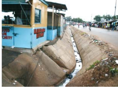
Waste gets into main drain
