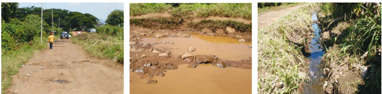
Fig. 2 Eroded earthen roads and trenches at some of the beaches
