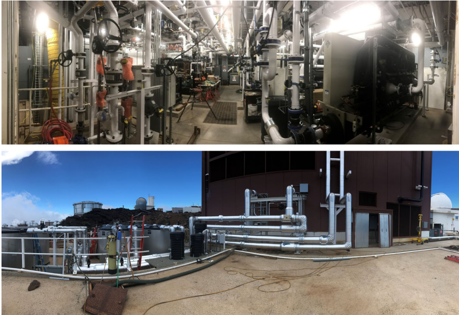
Figure 13 Inside of the utility building showing an example of the complex thermal systems infrastructure (top). Ice storage tanks next to the utility building (bottom). Also visible is the large dome structure of the AMOS telescope where the coating facility is located.
