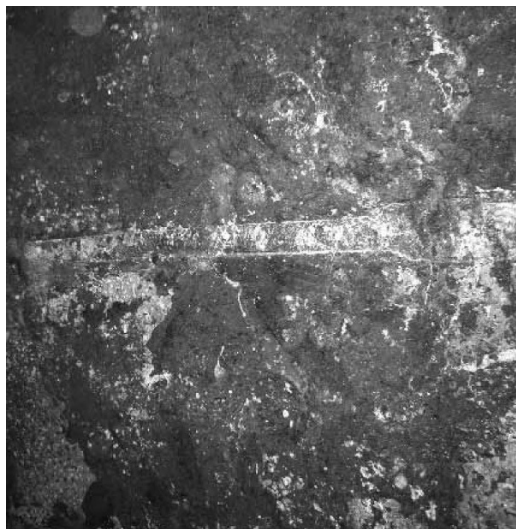
Fig. 4. Longitudinal cracks along hearth block.
