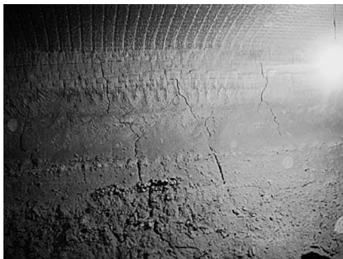
Fig. 4. Bank over rear wall.
