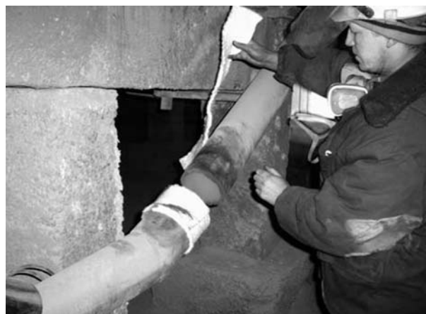
Fig. 5. Installation of Supersil S-10/140 in the insulation gap of the gas conduit beneath the body.
