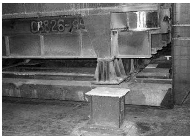
Fig. 4. Raised cathode unit with expansion fillers placed on the support of the unit.
