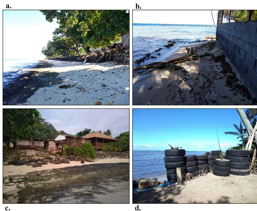
Fig. 2 Illustration of coastal armoring and erosion. a Beach rock exposure along the West coast of Moorea (Haapiti); b vertical concrete seawall in Moorea protecting a previously eroded plot of land; c level of income as source of varying coastal infrastructures; d home-made seawall made from old tires to prevent coastal erosion. © Maëlle Calandra and Jean Wencélius
