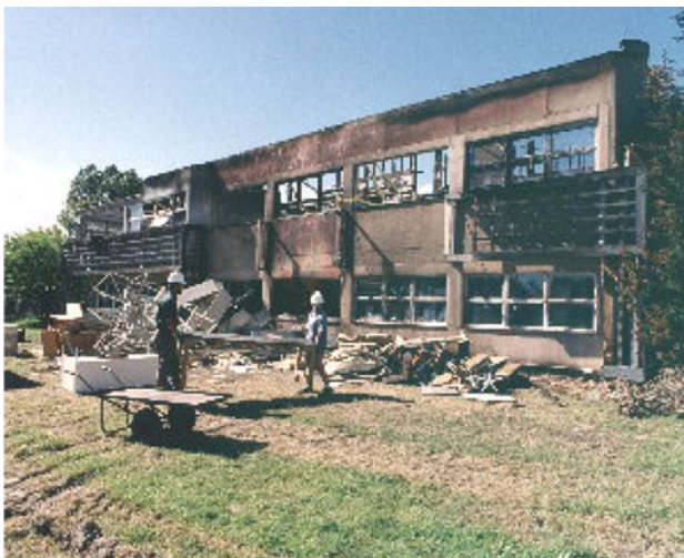
University Arson Fire: The fire bombing of Dr. Michael Podell's laboratory at OSU in 2001 caused extensive damage. OSU had employees and programs housed in the building
