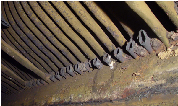
Fig. 5 Generating tubes in the superheater side
