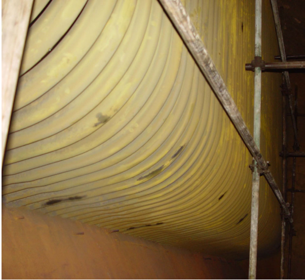
Fig. 4 Generating tubes in the economizer side
