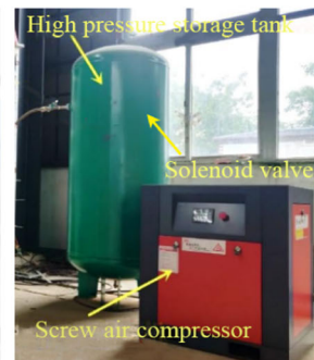
(e) Gas transportation system
