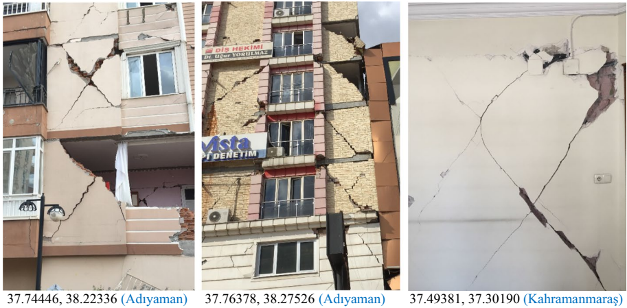
Fig. 30 In-plane damage to infill walls
