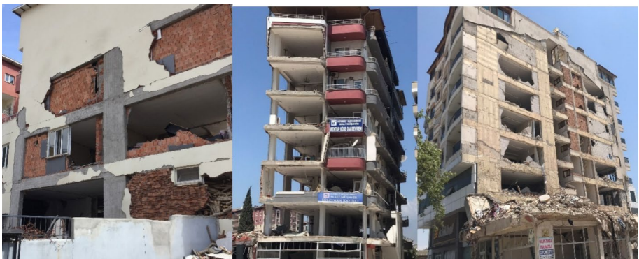
Fig. 31 Out-of-plane damages to infill walls
