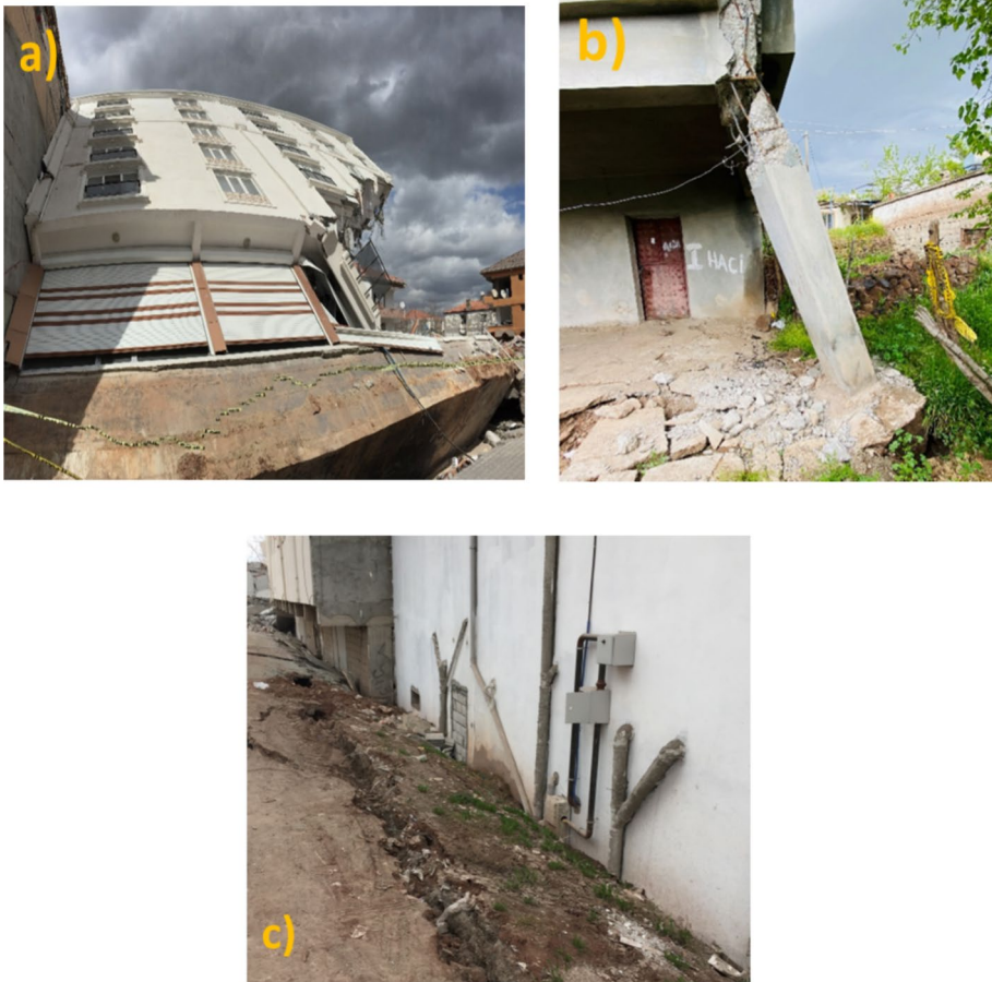
Fig. 32 Damages arose from the Soil and Foundation system
