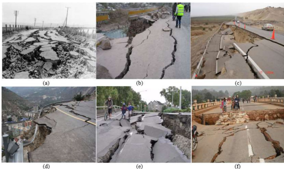
Fig. 1 (a) Damage to road in 1931 Napier Earthquake (Brabhaharan 2006) (b) Damage of road due to Muzaffarabad earthquake (Peiris and Free 2006) (c) Pan-American Highway damage near the Pacific Ocean due to Peru earthquake (O'Connor et al. 2007) (d) Road damage in Yingxiu due to Wenchuan earthquake (Zifa 2008) (e) Damaged road due to Christchurch earthquake (Anbazhagan et al. 2012) (f) Damage of bridge approach road due to Myanmar (Burma) earthquake 2001 (Anbazhagan et al. 2012)
