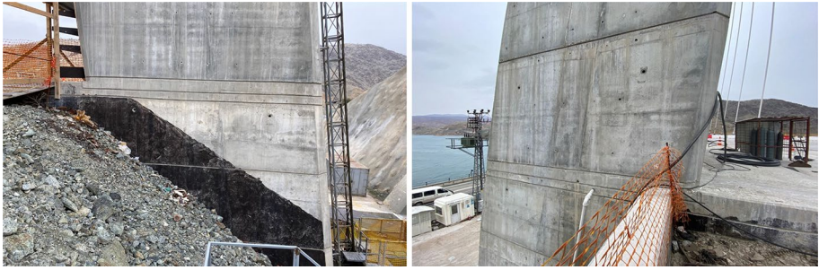
Fig. 7 Views from the foundation connection of the pylon on the Elazığ and Malatya sides
