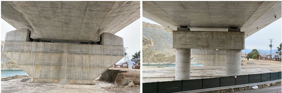
Fig. 8 Views from the shear keys, uplift points, supports, cap beams and piers
