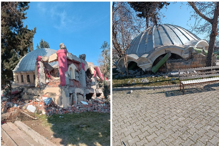
Fig. 37 The partial and total collapse of the mosque and its Shadirvan
