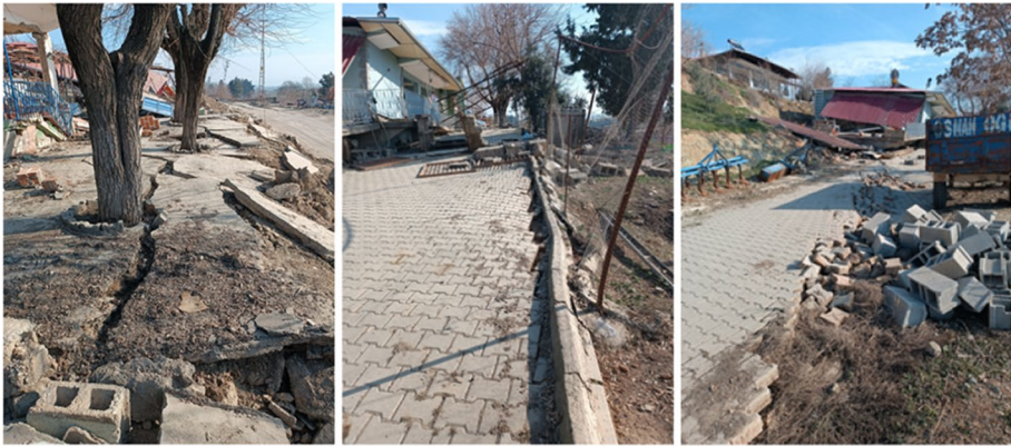
Fig. 10 Earthquake-induced surface damage in Kuyumcular village
