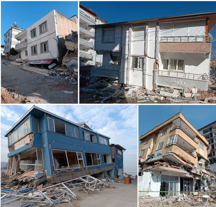
Fig. 13 Buildings collapsed as a result of soft/weak story mechanism
