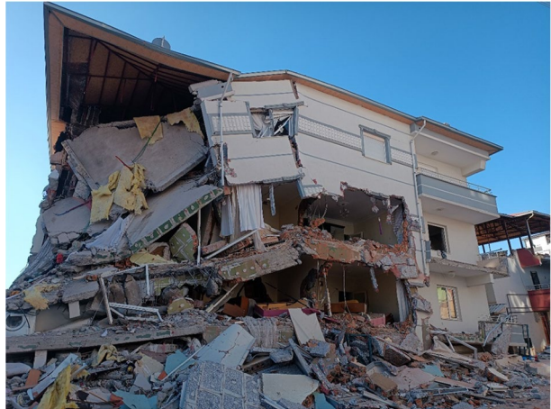
Fig. 17 The collapse of a part of the structure in the vertical direction
