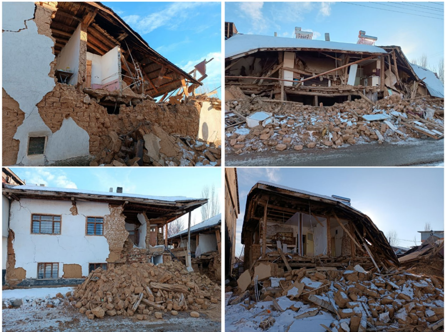
Fig. 27 Out-of-plane movement damages load-bearing walls
