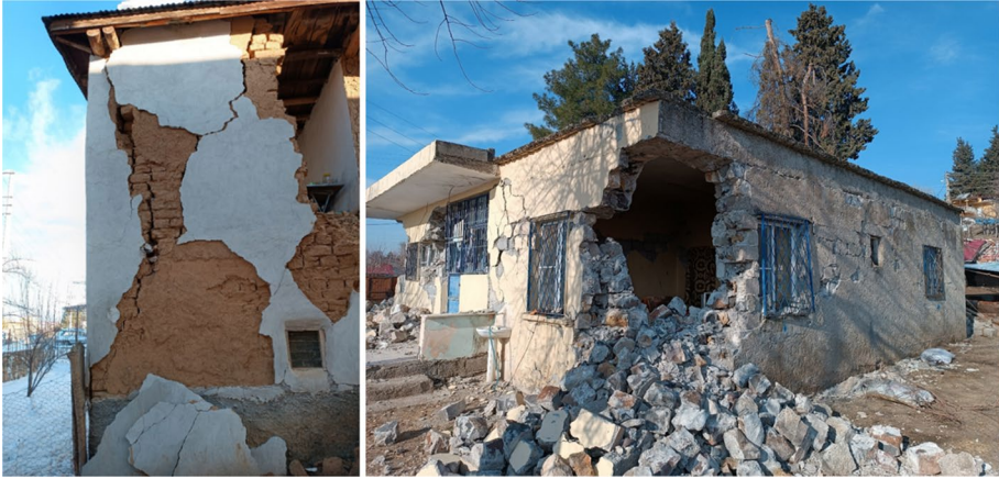
Fig. 28 Splitting damage at the wall corners
