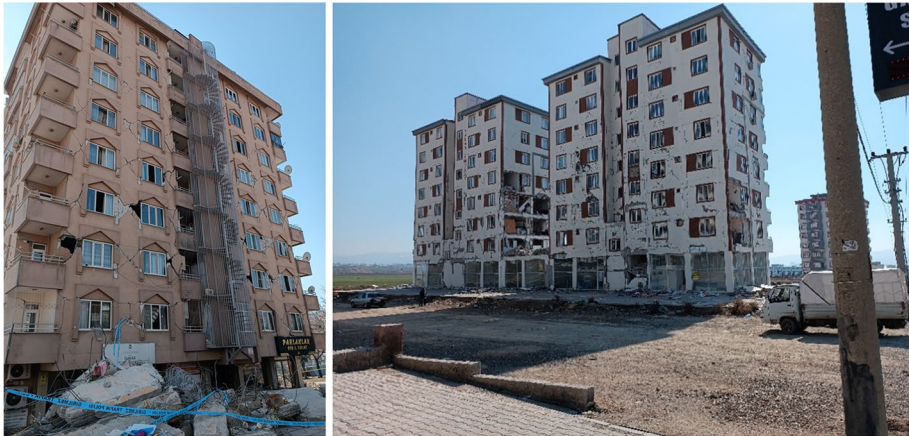
Fig. 20 Examples of infill wall damage
