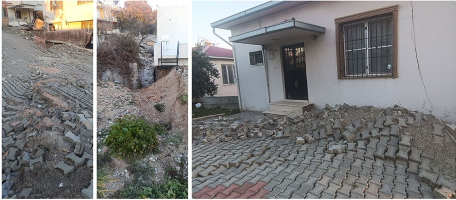
Fig. 9 Damages caused by the earthquake in Çiğli village center
