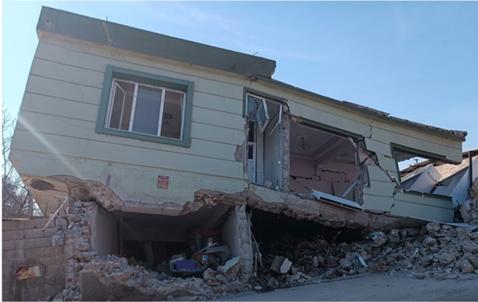
Fig. 30 Soft-story damage in a confined masonry structure
