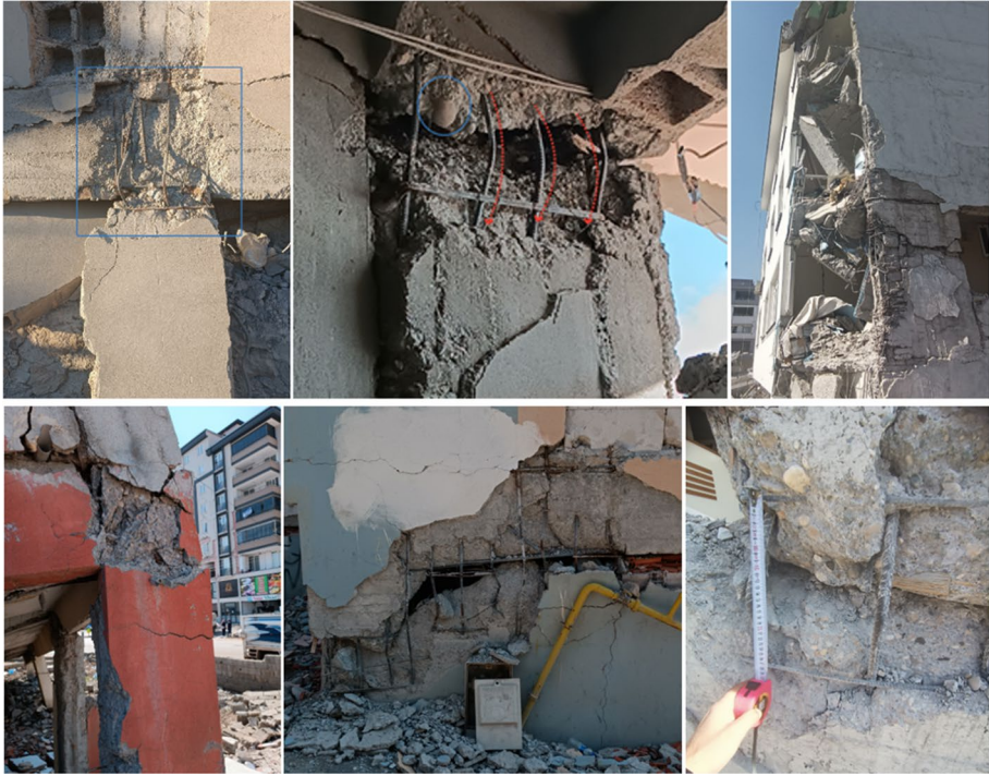
Fig. 22 Damages due to low-strength concrete and lack of reinforcement
