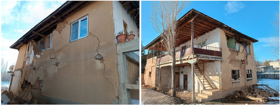
Fig. 26 Damages caused by window openings
