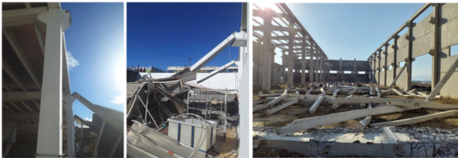
Fig. 33 Examples of industrial structures after the failure of the pinned beam-column connection
