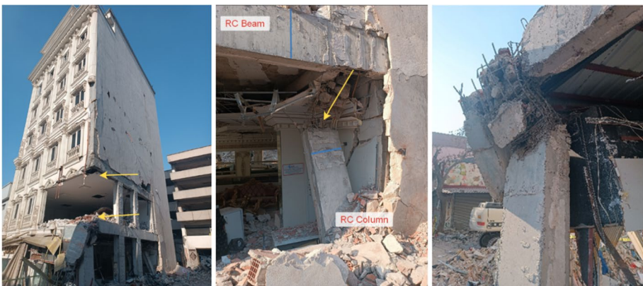
Fig. 15 Examples of RC columns heavily damaged by the impact of pounding
