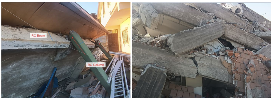
Fig. 21 Damages caused by strong beams and weak columns
