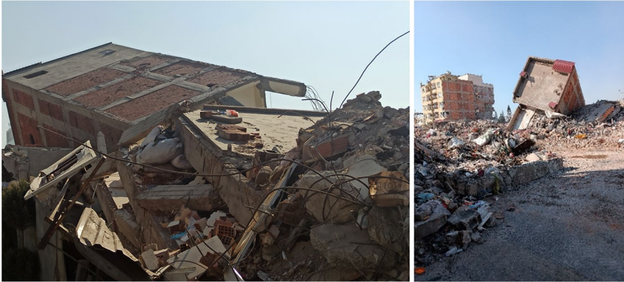
Fig. 16 Example of a building collapsing to the side
