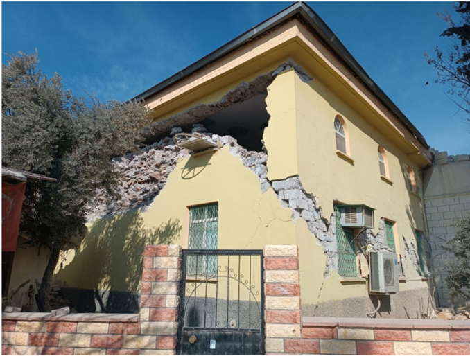
Fig. 29 Damages caused by the use of different wall materials and insufficient connection
