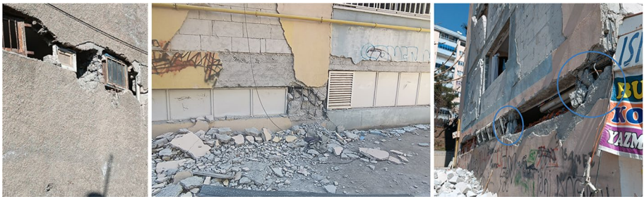
Fig. 19 Short column damages due to band-type windows
