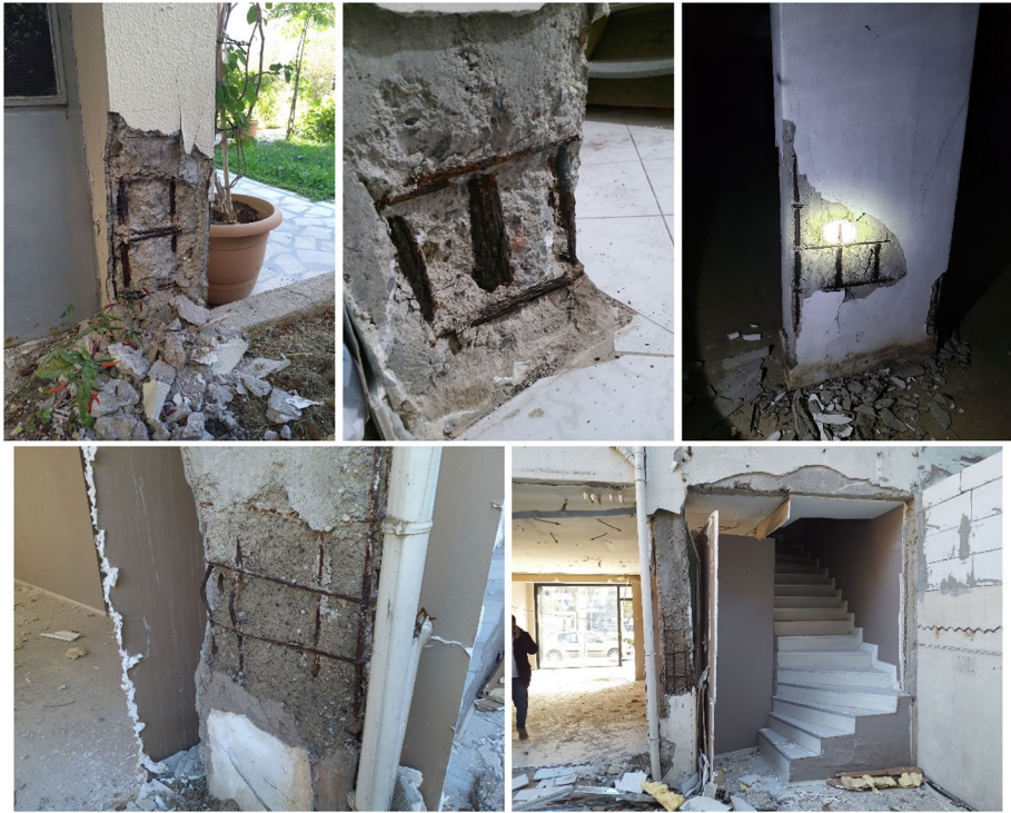
Fig. 20 Corrosion damages (image by authors and (AFAD 2021))
