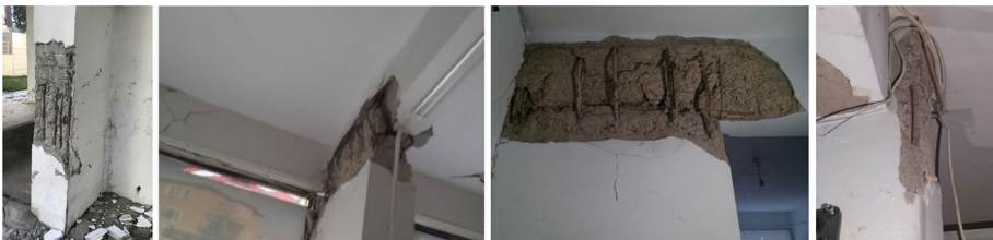
Fig. 13 Column-beam connection zone damages (image by authors and (AFAD 2021))
