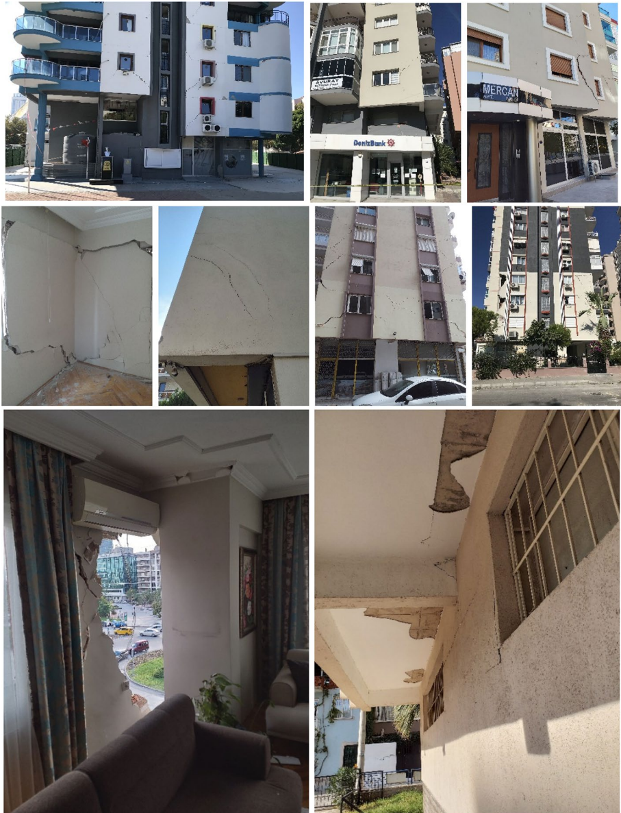
Fig. 16 Overhang damages (image by authors and (AFAD 2021))
