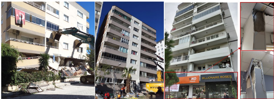
Fig. 9 The building examples damaged due to weak and soft story irregularity (image by authors and (AFAD 2021))
