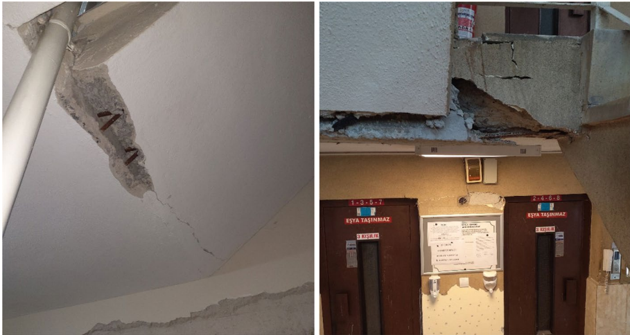
Fig. 18 Staircase damages (image by authors and (AFAD 2021))
