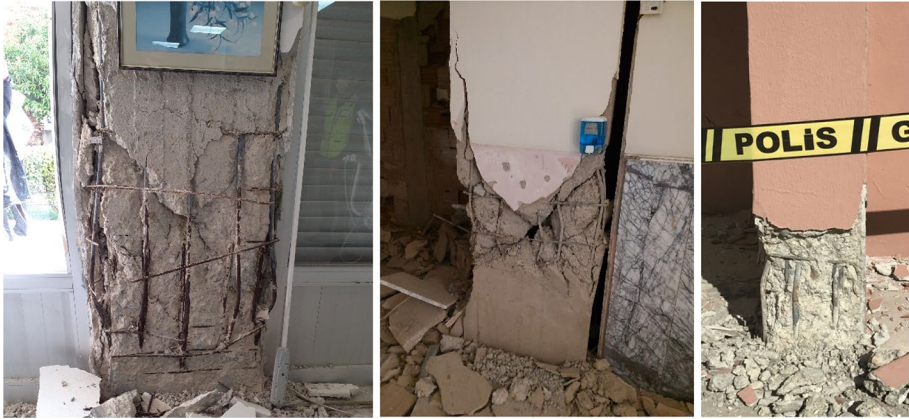
Fig. 11 Column damages (image by authors and (AFAD 2021))
