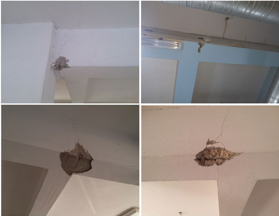
Fig. 17 Secondary beam damages (image by authors and (AFAD 2021))
