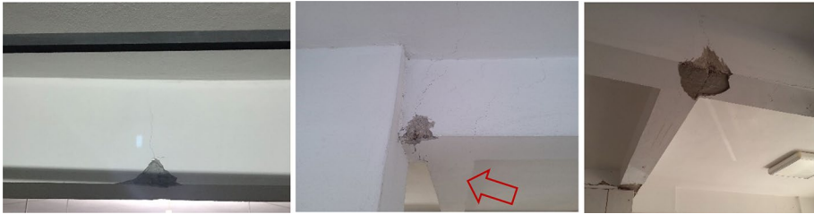
Fig. 12 Secondary beam damages (image by authors and (AFAD 2021))
