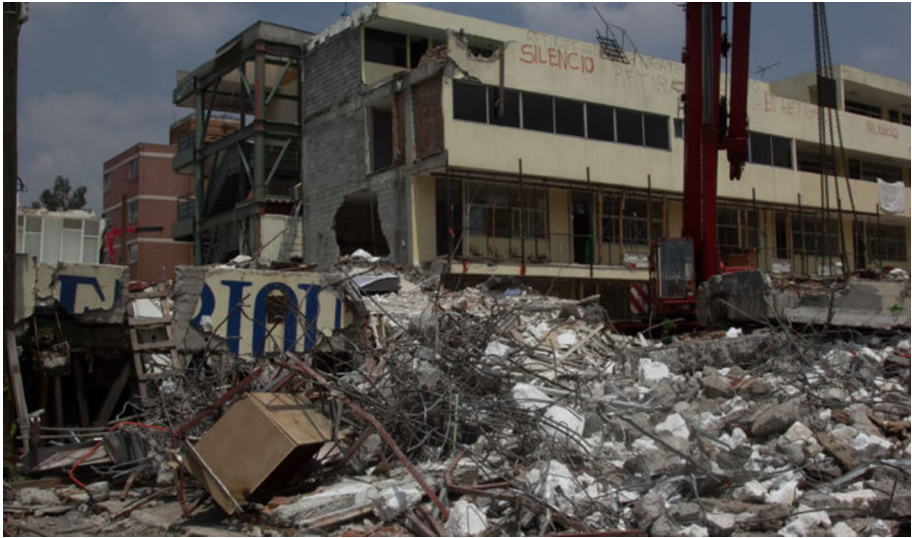
Fig. 3 The Enrique Rébsamen school, where 19 children and seven adults died in the collapse of part of the building during the EQKS19-2017 (Source: Animal Político, 2019)
