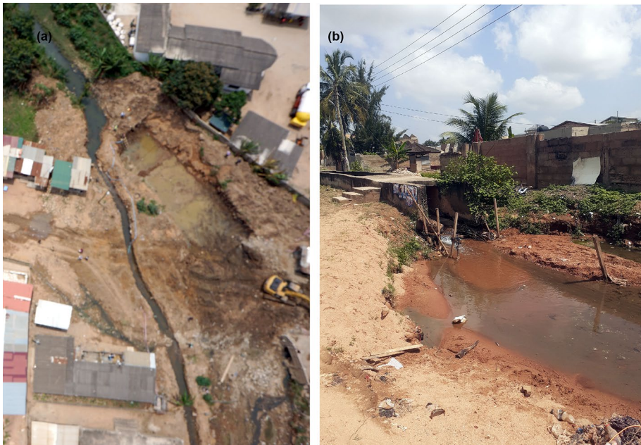
Fig. 14 a Aerial photograph capturing a location where a flood-prone bridge is enlarged, causing a bluespot with a considerable depth; and b evidence of erosion in a partial drain due to spillover from uphill areas
