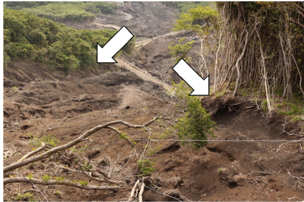
Fig. 18 Remaining parts of the disaster slope (view from the top)
