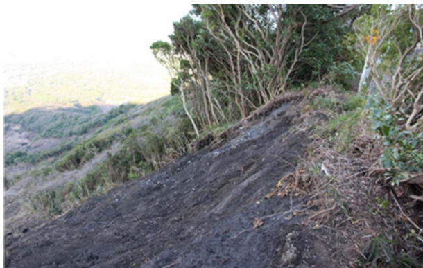
Fig. 6 Shallow shear failure at the initiation of slope instability
