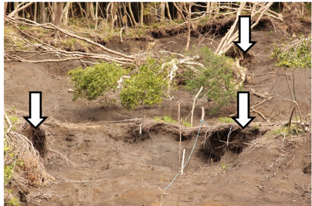
Fig. 9 Piping holes at the head scarp of the failed slope
