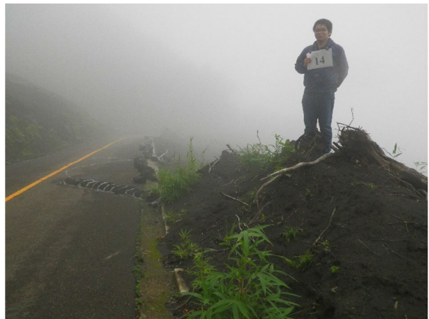
Fig. 22 Post-disaster situation at borehole site No. 14
