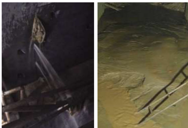
Fig. 6 Illustration of water ingress and mud inrush in metro system (Ren et al. 2016; Wang 2014)
