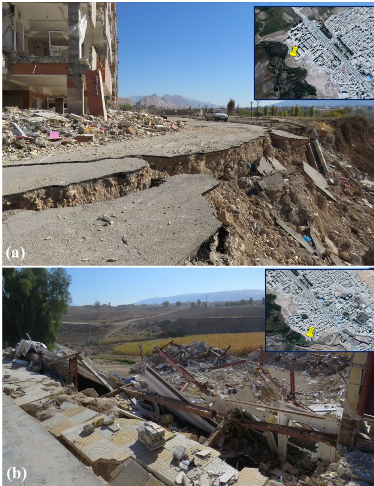
Fig. 2 The geotechnical aspect of the Sarpol-e Zahab earthquake a failure of soft soil embankment b collapse of the structure constructed on the weak ground
