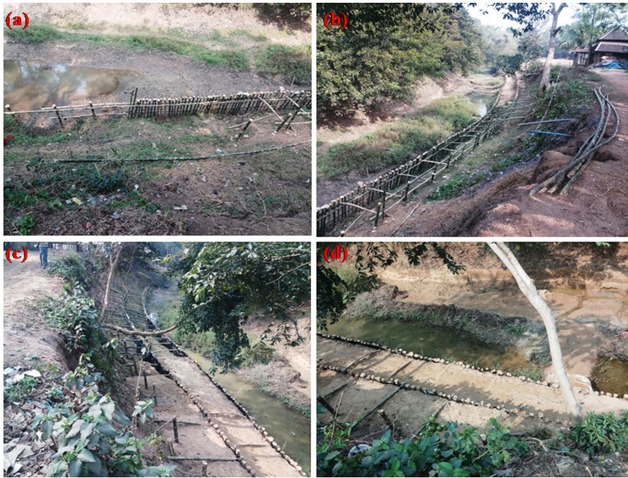
Fig. 3 Reach of the Ketia River at Shyampur village ( 22^{\circ} 36' 36'' N, 87^{\circ} 37' 33'' E), Ghatal Block, being prepared for planting the Vetiver buffer, a driving in of bamboo stakes, b aligning bamboo geogrids with bank geometry, c earth filling of the bamboo grids, and d a completed slope segment ready for transplantation
