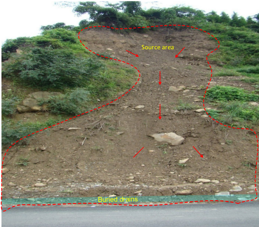
Fig. 4 A typical landslide along the highway
