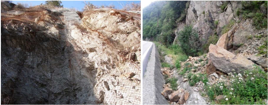
Fig. 10 Low-strength slope near Năruțu (left) and Brezoi (right), (SCS 2.00–3.00) (05.VII.2017)
