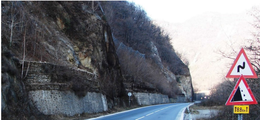
Fig. 23 Slope engineering works (high-tensile rockfall steelgrid mesh, dynamic rockfall berries, gabions, stone and concrete slabs walls)
