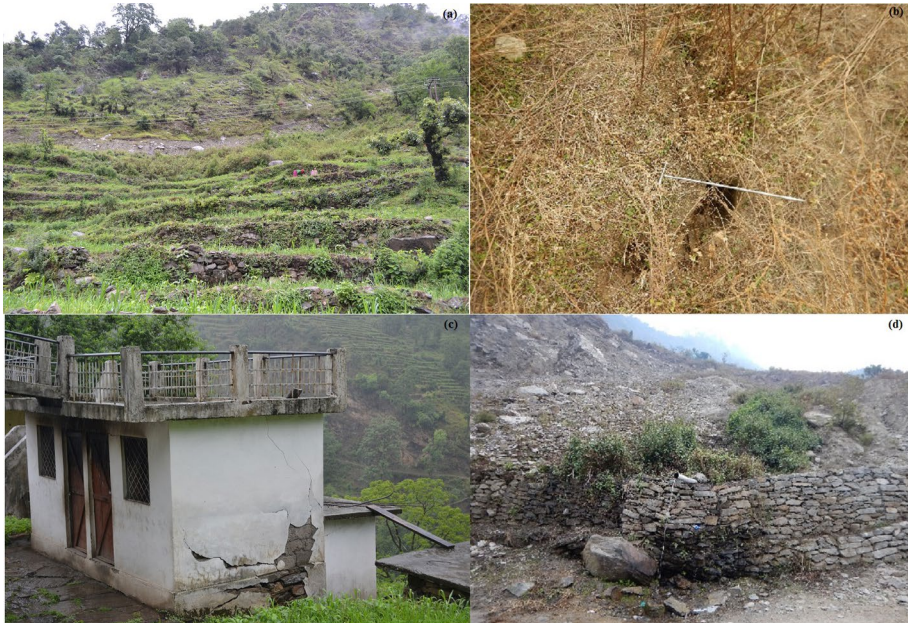
Fig. 7 a Developed scarp during 2013 extreme rainfall event of Kedarnath disaster, b tension cracks appeared on the unstable landmass, c damaged house which is located very close to crown of the landslide, d spring water along the flow path
