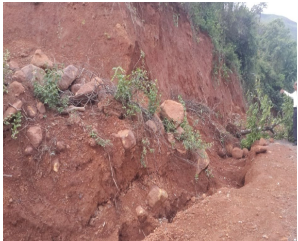
Fig. 4 Gully formation due to heavy rainfall
