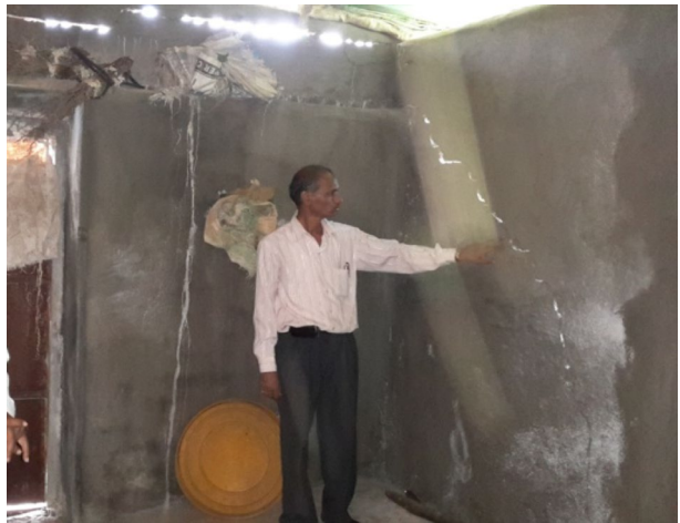
Fig. 6 Crack in wall due to settlement of foundation
