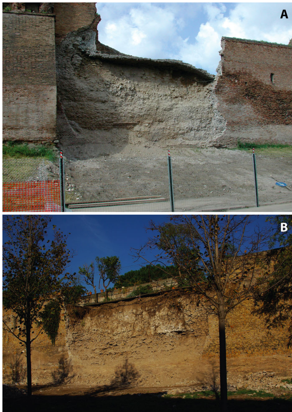
Fig. 16 Aurelian Walls of Rome: huge collapse due to ageing, lack of maintenance, and episodes of intense rain. a 16 April, 2001 (viale di Porta Ardeatina, southern sector of the Aurelian Walls); b 1 November, 2007 (viale Pretoriano, NE sector of the Aurelian Walls)
