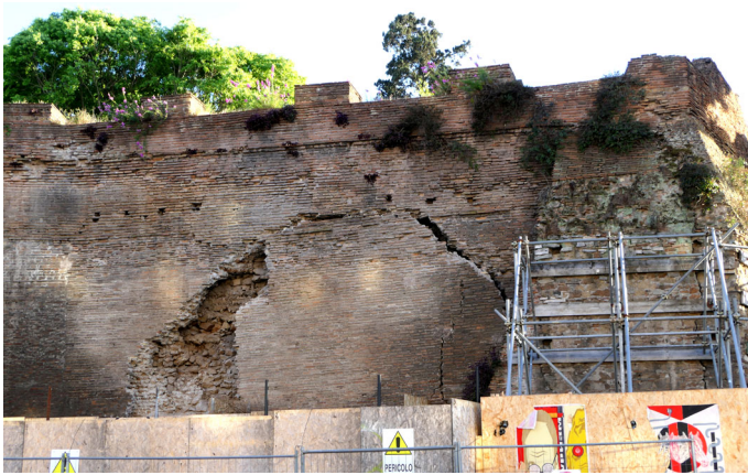
Fig. 17 Aurelian Walls of Rome: damage due to the earthquake (Mw 6.5) which originated in the central Apennines on October 30, 2016 (viale del Policlinico, northern sector of the Aurelian Walls)
