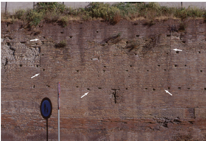
Fig. 7 Aurelian Walls of Rome close to Porta Pia: the sector indicated by the arrows has been attributed to a restoration subsequent to an earthquake that occurred during Late Antiquity (see text for further details)
