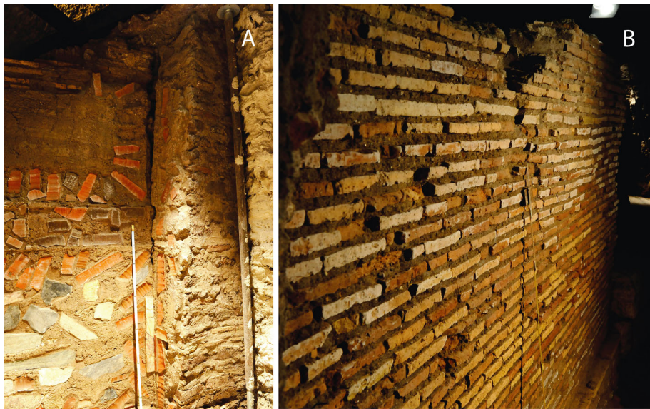
Fig. 5 Palazzo Valentini, domus B : a Open fracture in the eastern wall of the apsidal room. b Fissures in one of the perimetral walls of the domus , with the evident tendency for the toppling of the higher parts
