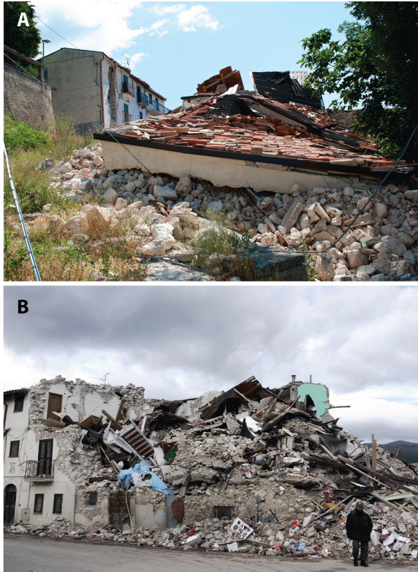
Fig. 10 Collapse of buildings due to the L'Aquila earthquake of April 6, 2009: a Castelnuovo: vertical collapse due to the excessive weight of the roof. b Onna: chaotic ruins lying over floors and the adjacent pavement
