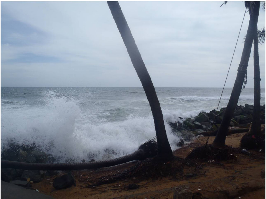
Fig. 16 Damages to seawall without frontal beaches at Bhimapally
