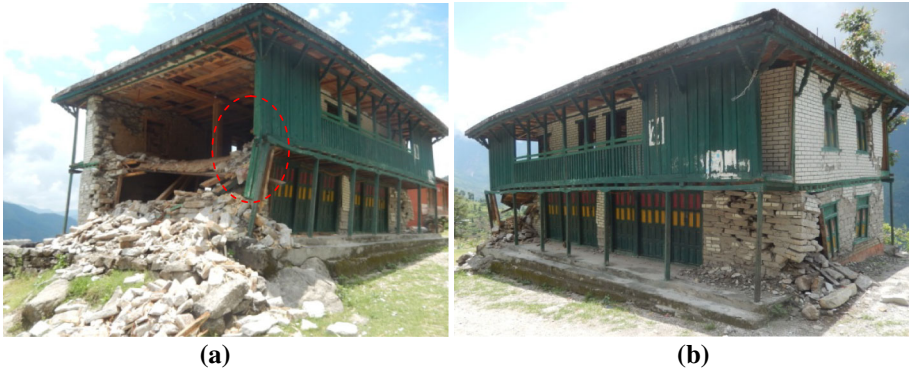
Fig. 19 Seismic damage to Thumo Gorka area due to landslide, rock falls and strong ground motion. a Out of plane collapse of masonry wall. b The view of the other corner
