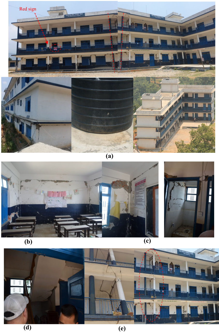
Fig. 8 Seismic damage to Shree Bandevi Secondary School. a Overview ( upper panels are connected at red dashed lines ). b The inner wall had light to moderate damage. c Crack between the window hole and the toilet door on the first floor. d Severe damages to the staircase connecting the first and second floor. e Large relative movement at the seismic joint. f The topographic map from the Google Earth
