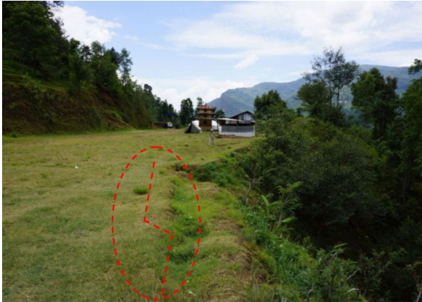
Fig. 27 Land rupture near the south cliff of the school (facing south)
