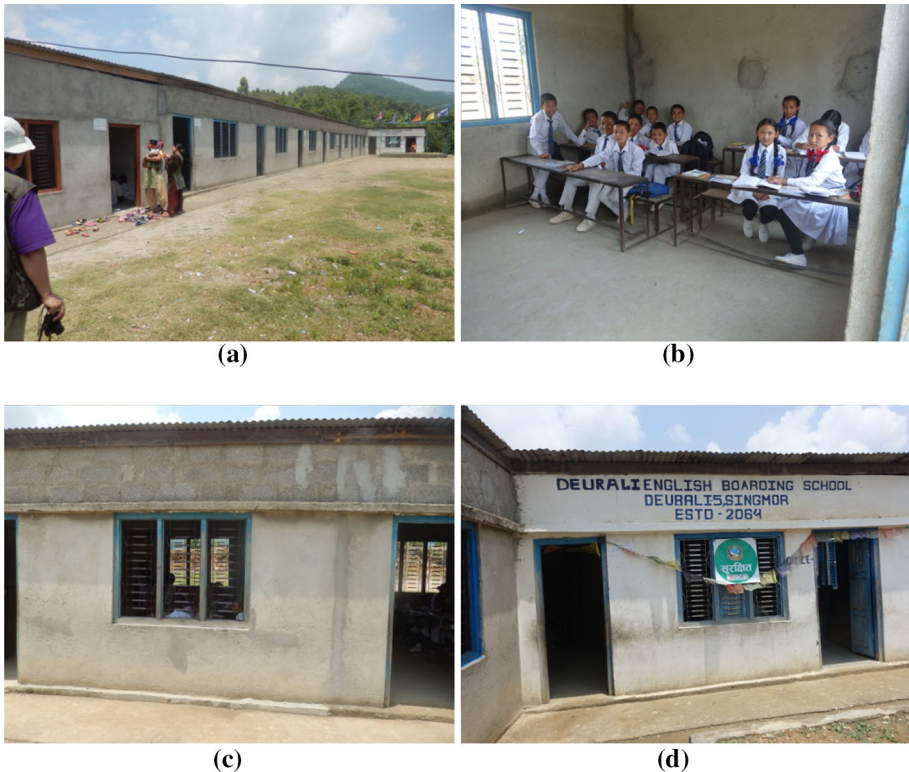
Fig. 16 Seismic damage to Deurali English Boarding School, constructed of light brick cement-bonded masonry. a Outside view. b Inside view. c Light brick over the heavy brick. d The school was verified to be safe as marked by the green sign
