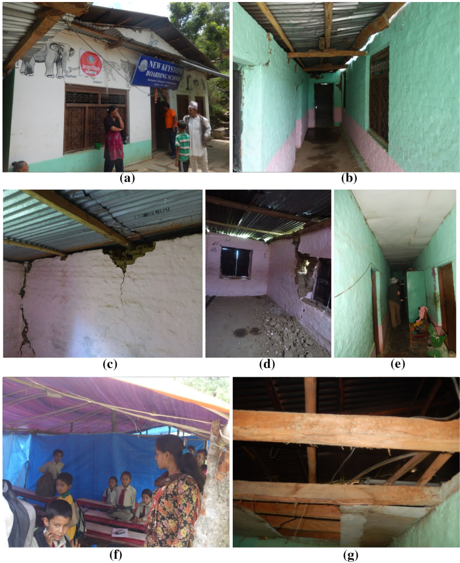
Fig. 17 Seismic damage to New Keystone Boarding School, constructed of low-strength cement-bonded masonry with simple timber frame roof with light corrugated plate. a School name. b The corridor. c Cracks of the wall under beam. d Severe cracks at the windows hole. e The corridor viewed from the opposite direction. f Temporary tents for teaching. g Electricity wires arranged around timber frame
