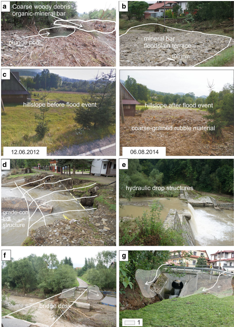
Fig. 6 Geomorphological changes of floodplain terrace (a, b, d) and hillslopes (c). Influence of hydrotechnical infrastructure such as grade-control (d) and hydraulic drop structures (e) on geomorphological changes of the river channel. Destruction of bridges (f) and culverts (g) as a result of erosional processes and organic material transportation. l —places where erosion occurred
