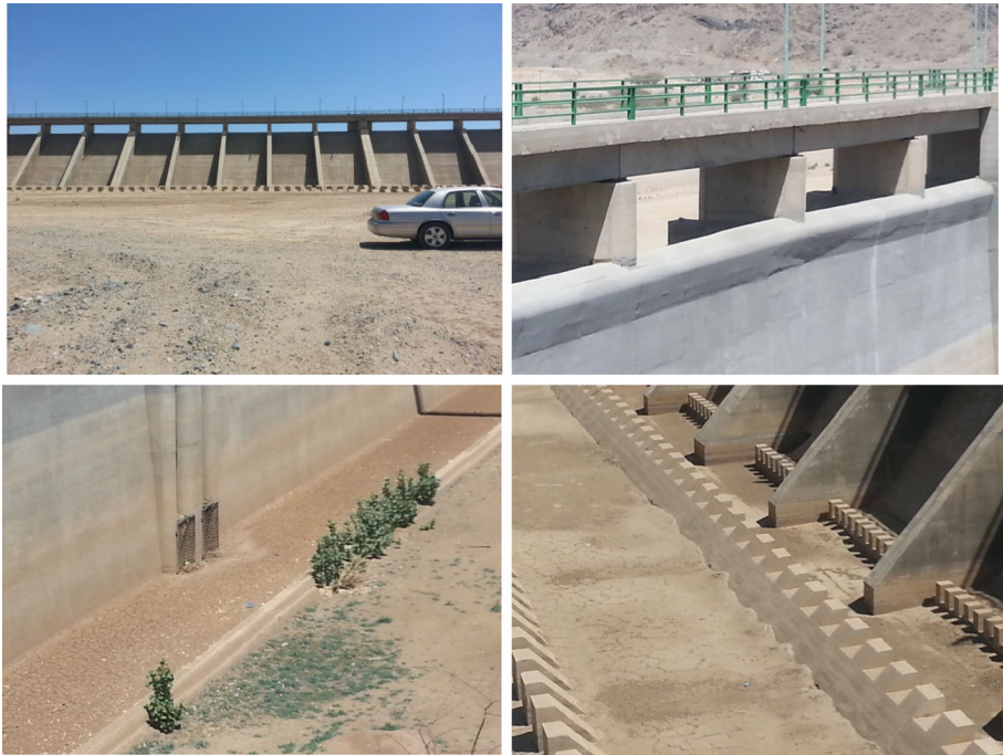
Fig. 7 Images of wadi Fatimah Dam: Top left (general dam view), top right (part of the dam spillway), bottom left (dam outlet looking from upstream) and bottom right (dam stilling basin with baffle blocks and end-danted sills)
