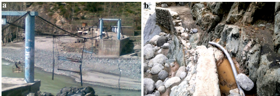
Fig. 6 a Damaged suspension bridge in the study area (photography by Shakeel Mahmood). b Damaged water supply scheme source in the study area (photography by Shakeel Mahmood)
