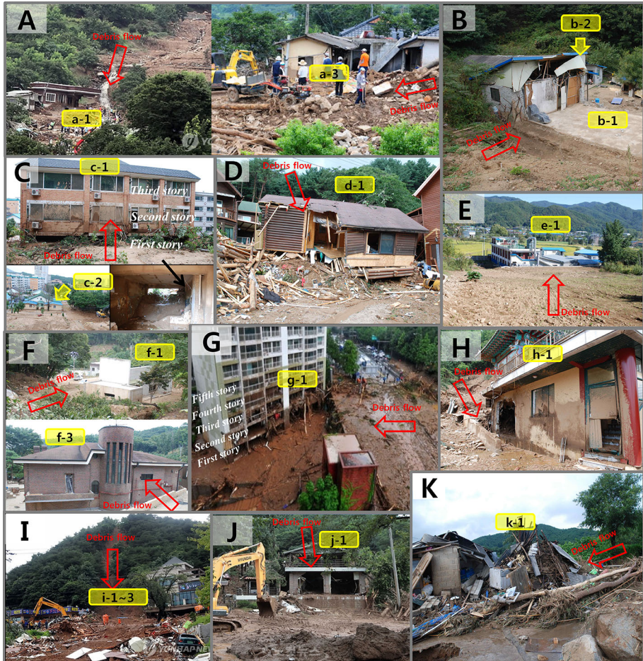
Fig. 6 Photographs showing buildings damaged due to debris flows in a Miryang, b Yongin, c Pocheon I, d Pocheon S, e Dongducheon H, f Gwacheon, g Seocho, h Dongducheon S, i Chuncheon I, j Chuncheon J, and k Jeongseup
