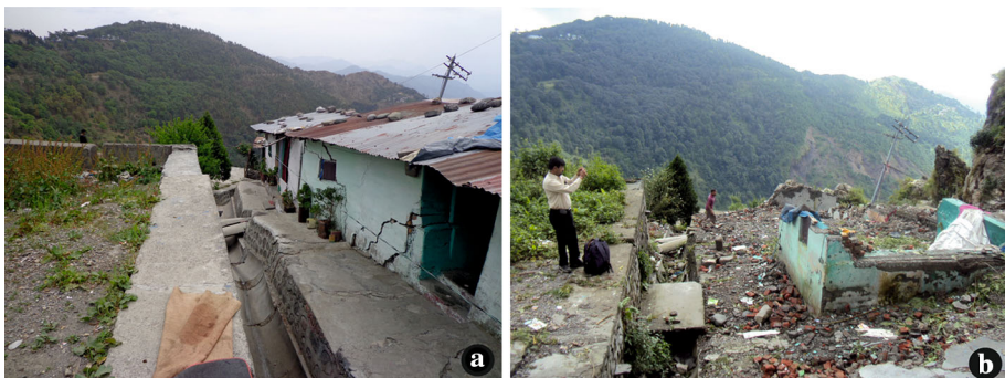
Fig. 4 a Cracks on the walls of the houses located adjacent to the GIC playground before the occurrence of September 2014 Rais Hotel colony landslide and b subsidence of the area and damage to the houses after the occurrence of September 2014 Rais Hotel colony landslide
