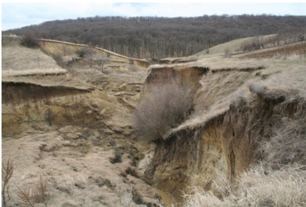
Fig. 6 Active landslides in the lower reach of Valea Adanca Gully, Puriceni Gully system (April 01, 2012)
