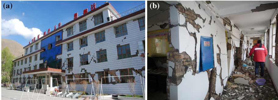
Fig. 16 X-shaped cracks in bearing walls and cracked and partially destroyed interior longitudinal walls in an office building of a police station constructed without columns and belt courses (Part I)
