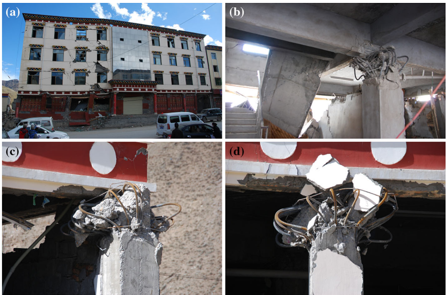
Fig. 12 A four-story RC frame building near Shangye Road and Baqu River with yielded column ends in the soft first story and cracked infill walls around some upper floor windows (Part IV)
