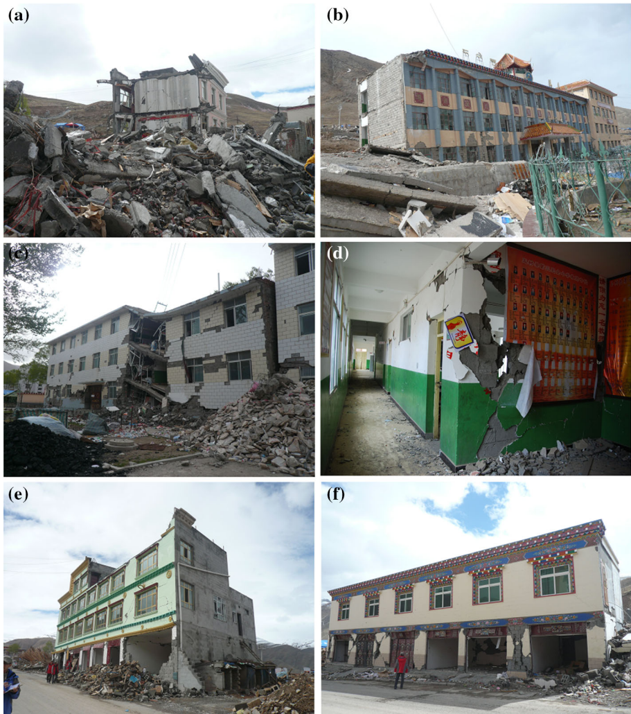
Fig. 7 a A completely collapsed concrete block building near South Xihang Road (Part II), b an extensively damaged teaching building in a college (Part III), c an extensively damaged male-student dormitory building at a college (Part III), d partially destroyed bearing wall on the first floor of an elementary school building (Part III), e partially collapsed and cracked bearing walls of a concrete block building near North Xihang Road (Part II), f cracked bearing walls at the first story of a concrete block building near West Xihang Road (Part II)
