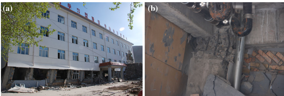
Fig. 10 A tilting RC frame building of a police station with yielded column ends on the soft first floor and cracked, partially destroyed infill walls (Part I)
