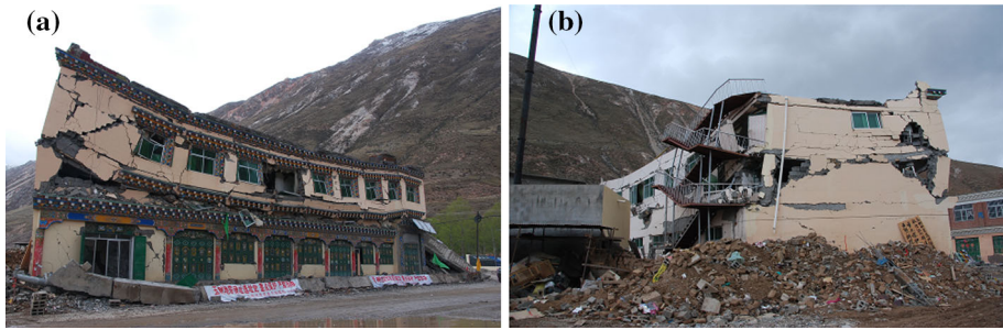
Fig. 19 Collapsed second floor that was used as a large restaurant in the Gesaer Hotel building (Part I)
