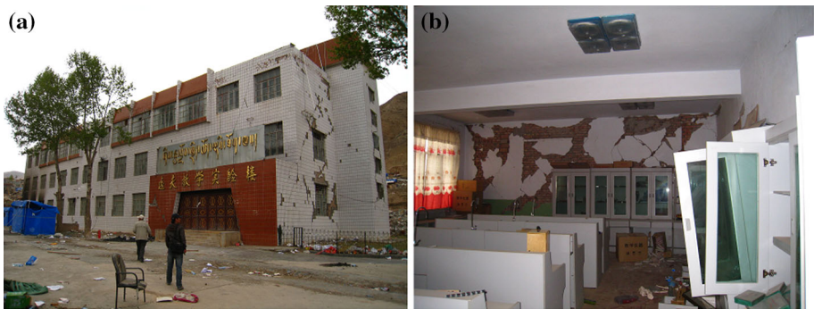
Fig. 15 A building in a college with X-shaped cracks in bearing walls and severe damage to interior walls (Part III)
