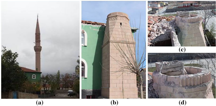
Fig. 4 Minaret at Helvadere Village collapsed from the above of transition segment. a Formerly taken photograph (URL-2 2013), b remained parts, c and d transition segment and reinforced concrete inner stairs
