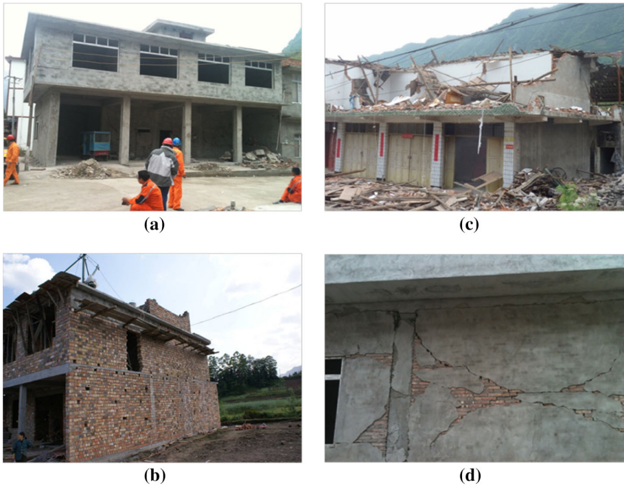
Fig. 9 Typical rural house structures and consequent damage
