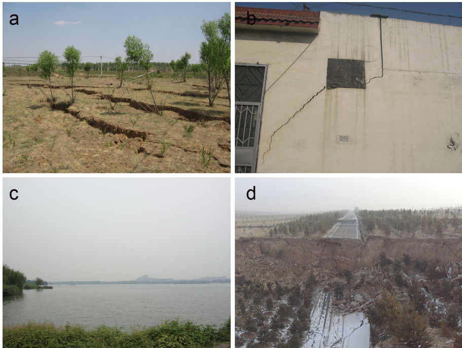
Fig. 1 Environmental problems and/or hazards induced by surface subsidence. a Landscape modification in Daliuta coal mine in Shendoing mining district (occurred in 2009), b building damage associated with Xuchang coal mine in Zibo mining district (occurred in 2004), c waterlogging in farmland surrounding Yangzhuang coal mine in Huaibei mining district (occurred before 2005) and d road damage above Taian coal mine in Yangquan mining district (occurred in 2011)
