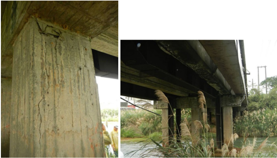
Fig. 1 Chloride-induced corrosion in an RC bridge
