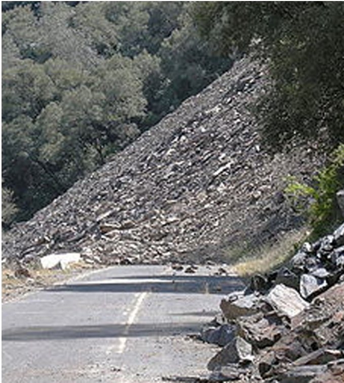
Fig. 8 Heavy landsliding on Chakothi Road
